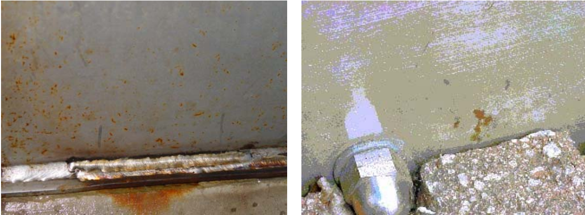
Fig 7. Grade 4404 (316L) stainless steel contaminated with carbon steel during installation.
