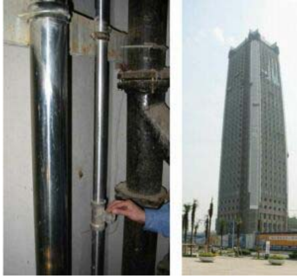
Figure 6. Plumbing system in new telecommunications building in Xi'an, China.
