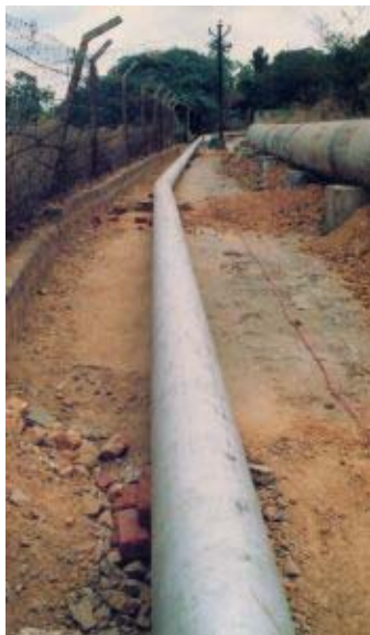
Figure 1. The first use of a stainless steel pipe to handle raw water in India. 300 mm diameter: lower weight meant lower transport and installation costs; no corrosion meant that pumping efficiency would be maintained. Compared with
