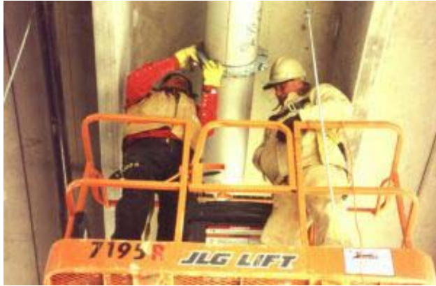
Figure 3. 300 mm drinking water main pipe, light enough to be installed by two people in a new sports stadium in Detroit, USA.
