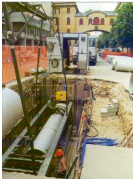
Figure 5. Refurbishment of water main in Padua, Italy using trenchless technology to avoid disruption. Lengths of pipe are orbital welded in the excavation and then pushed hydraulically along the old main.
