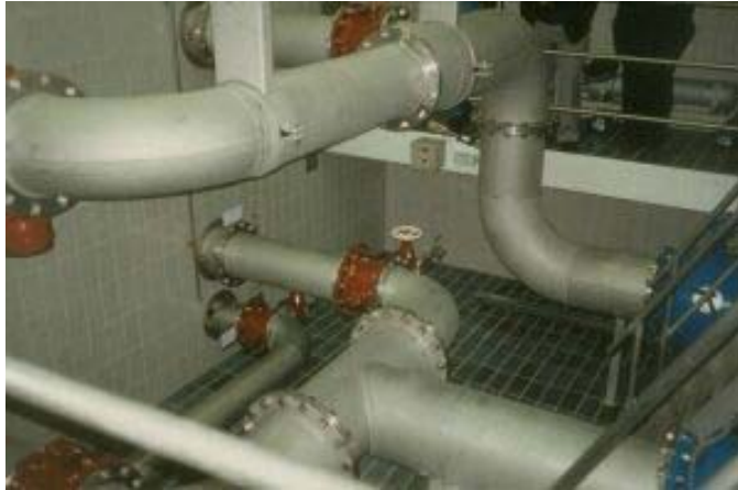
Figure 8. High standard of fabrication of pipework in a drinking water treatment works, Germany.
